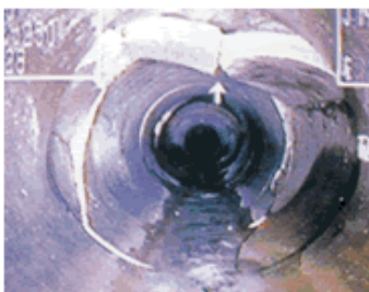
Inside of a collapsed pipe
